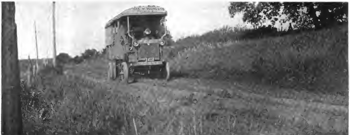
This gumbo road has been scraped and a slight attempt made at crowning, but has no side drains. Rain cannot readily run off and the surface becomes treacherous. Too much attention to width has not only cut down the work on the first making, but also presents quick dragging after rain
